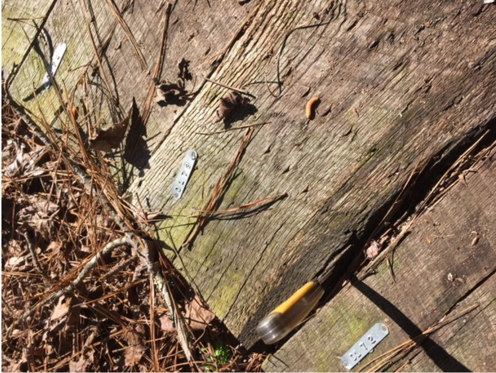
Figure 2 - Tie #173 with light decay.
