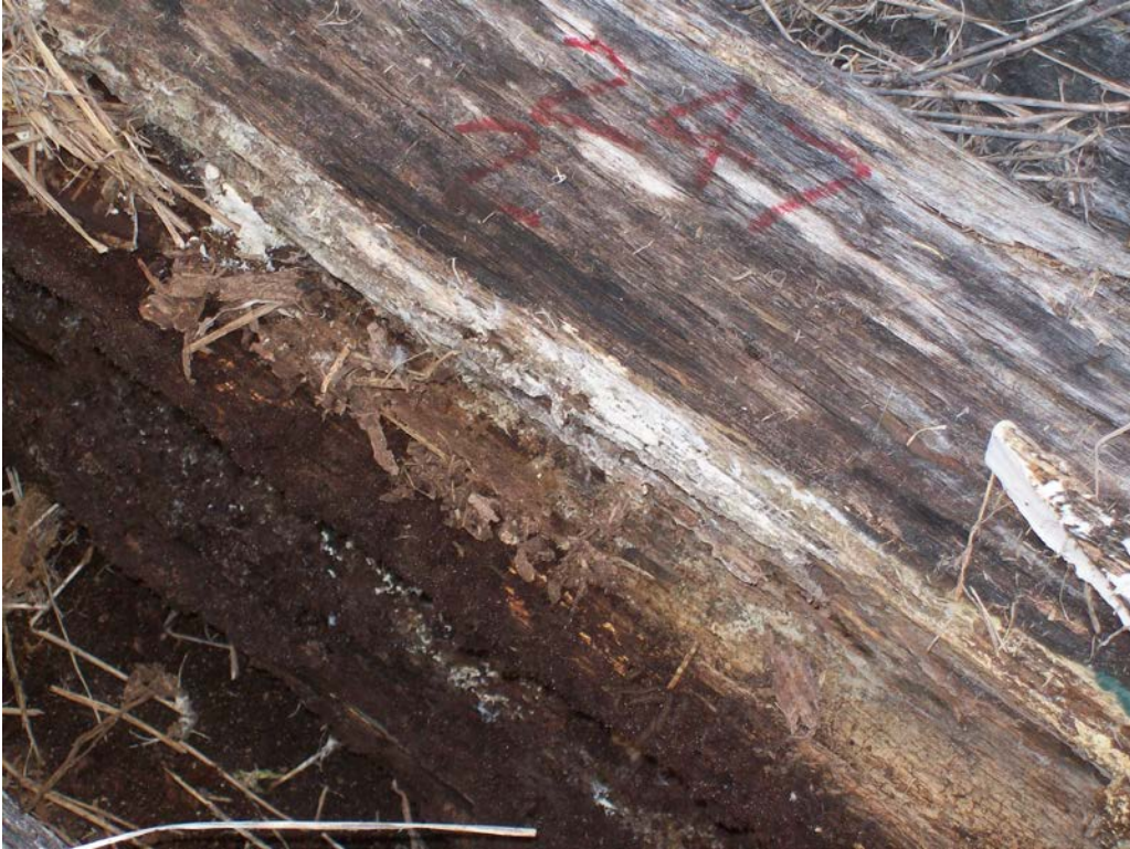
Figure 8 - Tie #247 with severe decay and trace termite damage.
