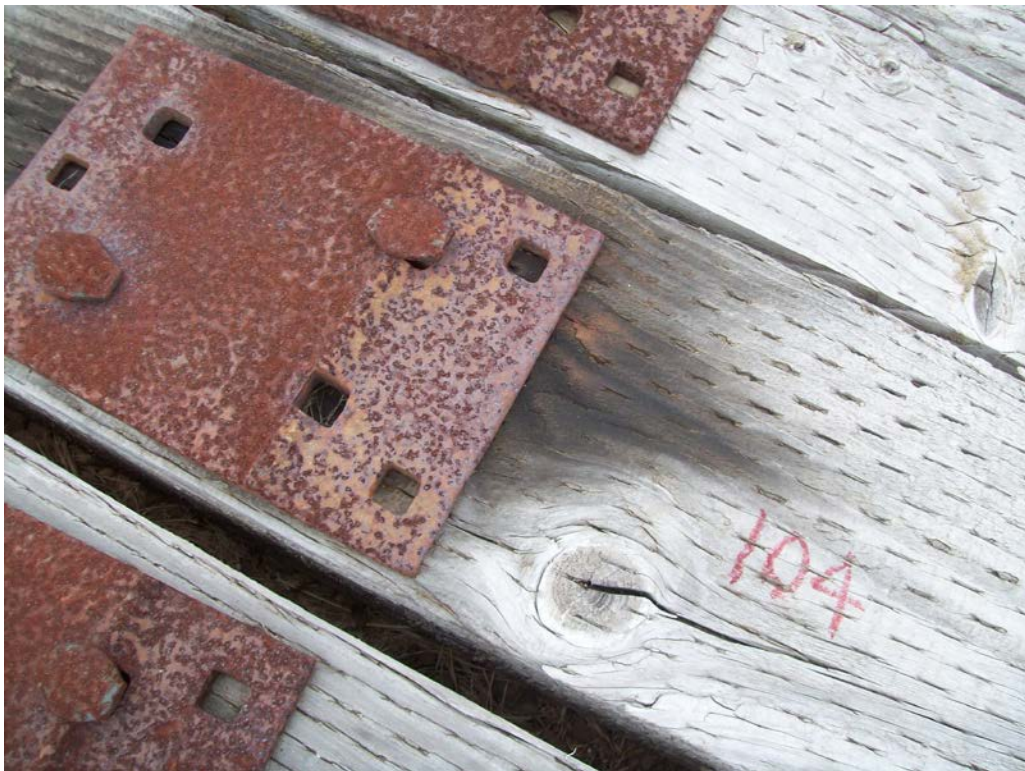
Figure 7 - Tie #104 with "iron stain".
