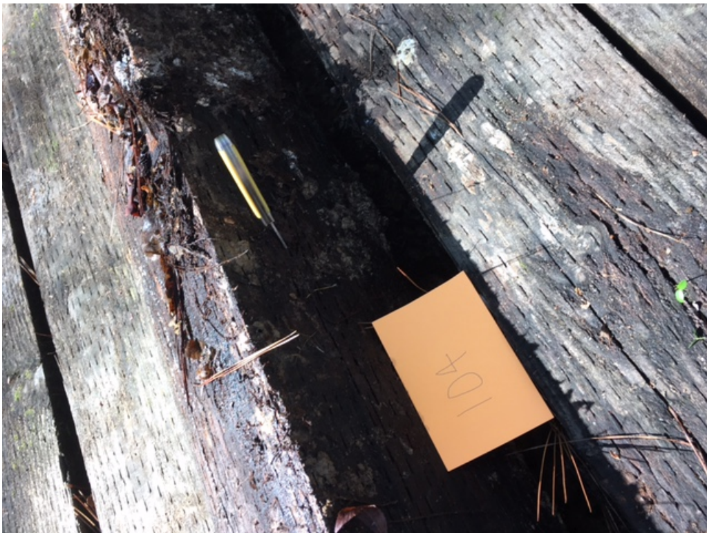
Figure 3 - Tie #104 with decay and trace termite damage.
