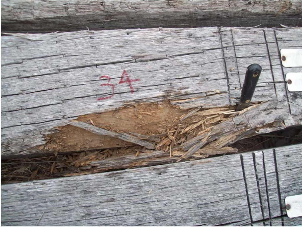
Figure 6 - Tie #34 with decay and slight termite damage.
